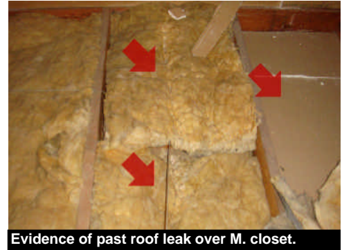
Evidence of past roof leak over M. closet.
