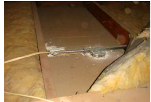
Unsecured ceiling fan wiring.
