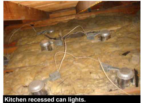
Kitchen recessed can lights.
