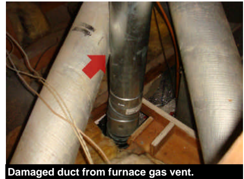
Damaged duct from furnace gas vent.
