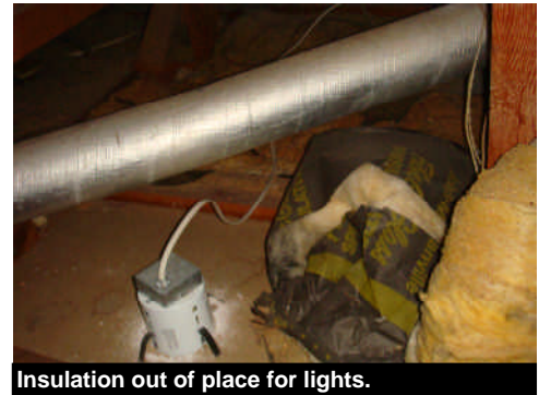
Insulation out of place for lights.
