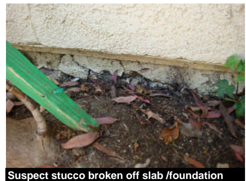
Suspect stucco broken off slab /foundation
