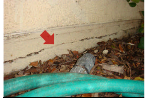
Cold joint between foundation & slab.
