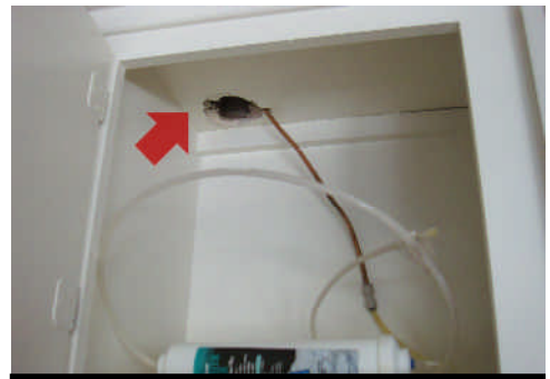
Hole in the ceiling, and unsecured line.
