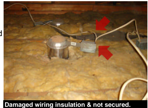
Damaged wiring insulation & not secured.
