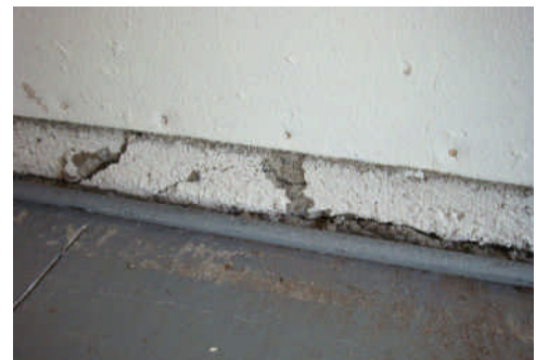
Garage broken concrete foundation /slab.
