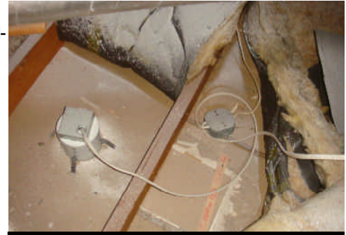
Unsecured wiring and junction box.
