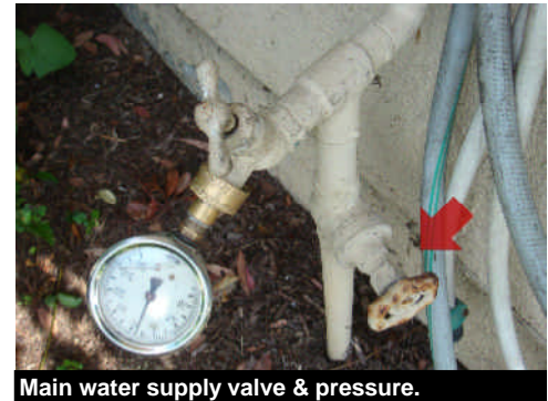
Main water supply valve & pressure.
